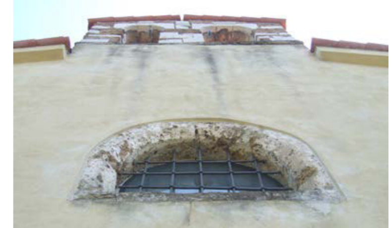
Vaulted window frame made of the local travertine, in the church at Dolina
