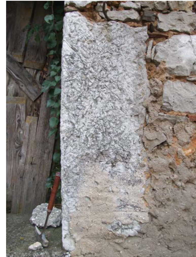
A poor quality stone frame made from local Alveolinid-numulitid limestone (Grozžana/Gročana)
