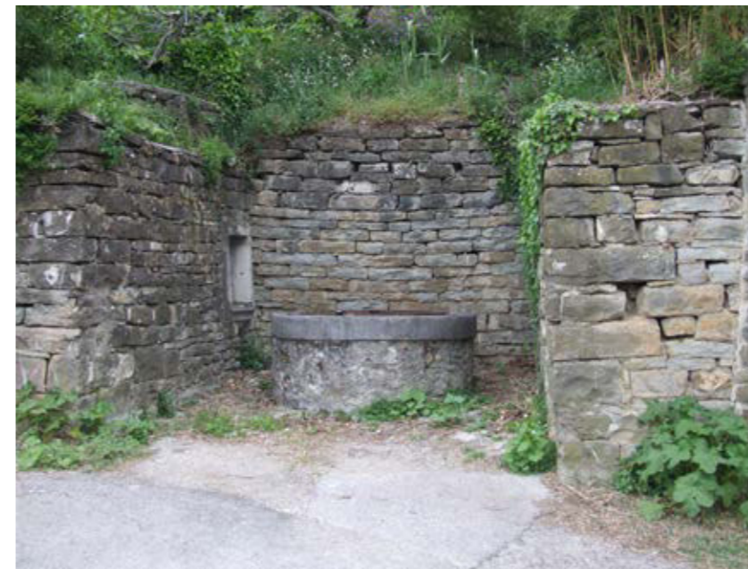
Fresh (not weathered) greyish-green sandstone blocks are a reliable indicator that flysch blocks originate from a quarry, dug out from deeper layers (Prebenico/Prebeneg)
