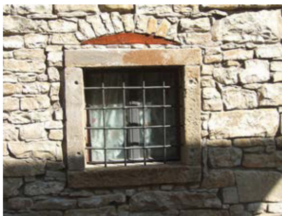
A window reveal of Cretaceous limestone. Above it is a load bearing arch of flysch sandstone, with a timber load bearing element beneath it
