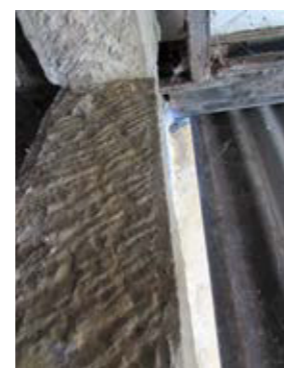
Roughly treated flysch sandstone door frame
