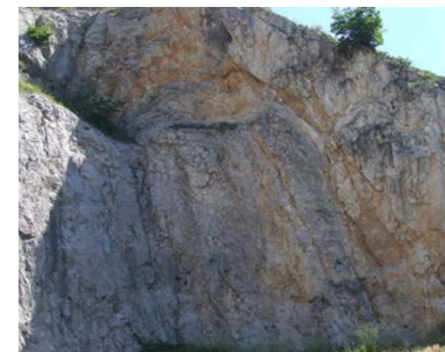
Alveolinid-numulitid limestone in the Scoria quarry above San Giuseppe della Chiusa/Ricmanje unsuitable for stonemasonry due to intense fracturing, despite the bedding in the quarry exhibiting no large displacements
