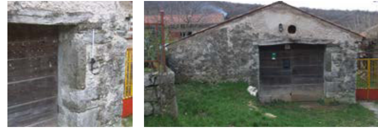
Side framing of a gate built of larger blocks of local limestone and flysch sandstone. The lintel is timber because local stones lack suitable mechanical properties
