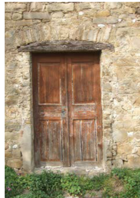
Timber lintel over a gate. Above it is a load bearing stone arch of flysch sandstone building blocks
