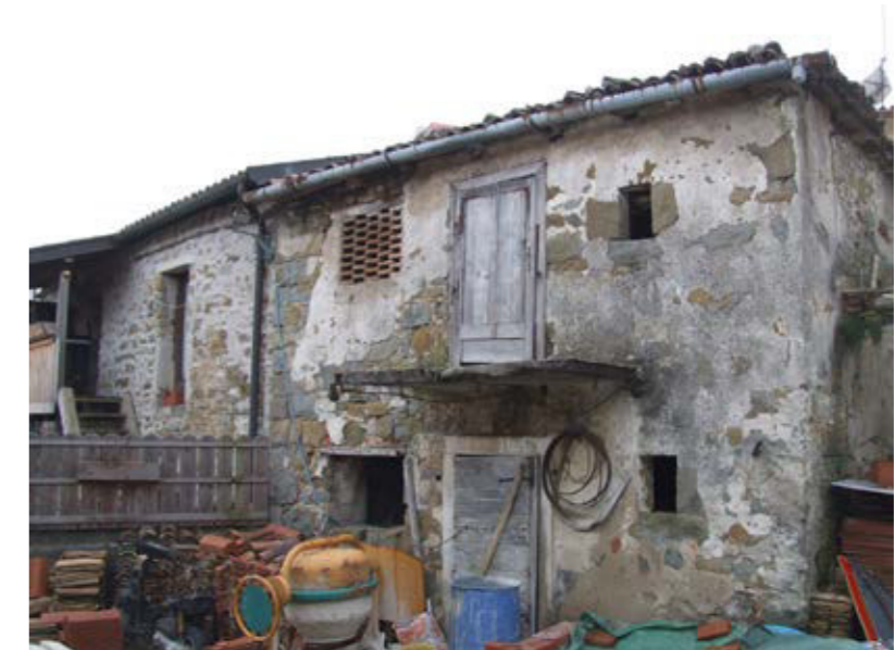
A row of buildings with a distressed cantilever balcony
