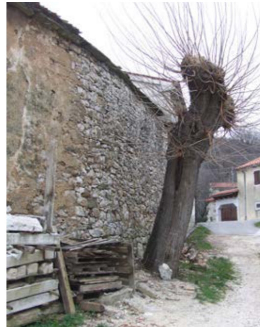
A typical frontage blanked in the direction of the Bora wind. As a rule, outside walls were rendered, as there was plenty of material for limestone plaster in the vicinity. Since local construction materials are of a poorer quality prone to dissolution and erosion, rendering façades is a reasonable measure to extend the life of buildings constructed with local stone, while also taking into account all other characteristics and qualities of existing walls and given sound selection of materials and plaster making techniques. Note the mulberry tree by the wall. Mulberry trees in the Karst communities and substantial parts of Breg recall a time when silkworm rearing was a local business
