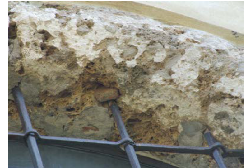
The vaulted window frame was completely covered in plaster and painted
