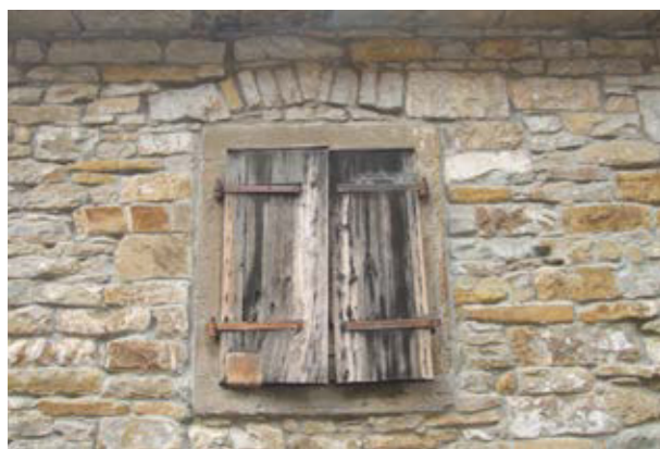
A window frame of flysch sandstone with a load bearing arch also of flysch sandstone. Note the traditional full shutters
