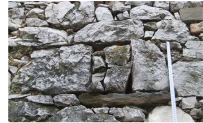
A typical window reveal with side stays and a lintel of local limestone. The sill is of flysch sandstone. The shape and size of the window is typical of an earlier period predating stone treatment techniques that emerged in the 18th and 19th Centuries. Window reveal sizes depended on the local limestone which has relatively low natural compressive and flexural strength. Technical advances and lifestyle changes brought larger reveals, the trend enduring to this day
