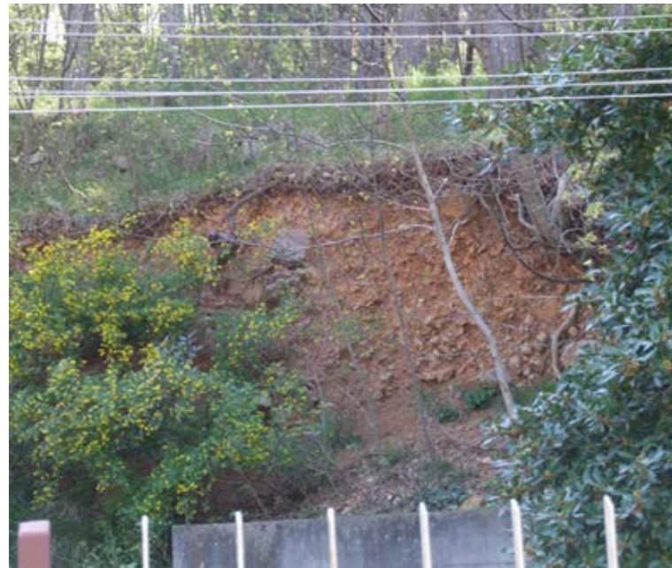
Slope limestone gravel with sandy silt and sandstone clasts from weathered flysch (Dolina)
