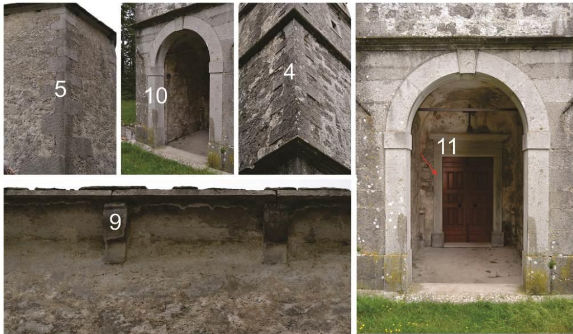
Parts of the building (elements): 4-bell tower corner stones, 5-church corner stones, 9-flared portion corbels, 10-bell tower vault, 11-main door doorpost
