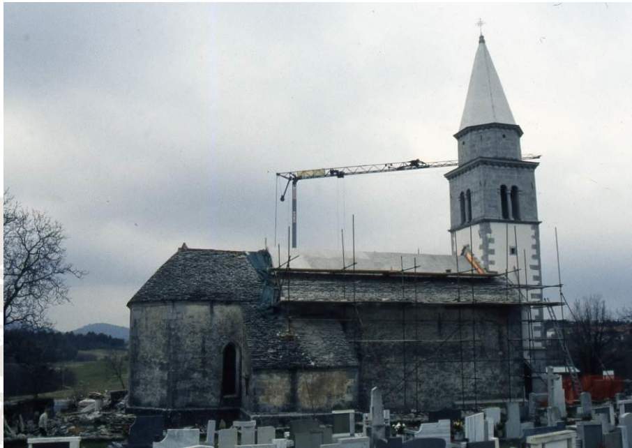
Figure 5.17 Renovation of the roof on the church in Križ village. Originally it was roofed using Tomaj limestone, which was partly replaced by the fractured limestone from the Lipica Fm. (archive photo, B. Jurkovšek).
