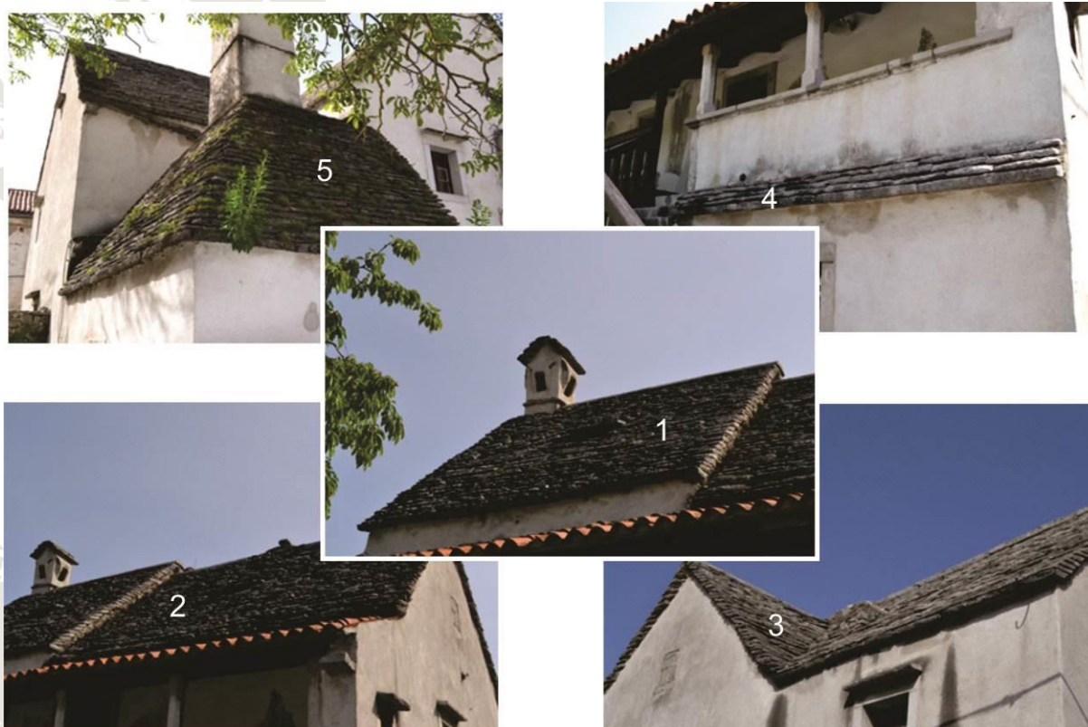
Parts of the building (elements): 1-main roof (South) W part, 2-main roof (South) E part, 3-main roof (East), 4-small roof along stairs, 5-extended kitchen roof
