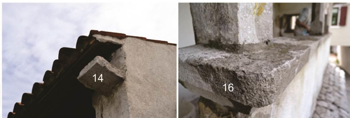
Parts of the building (elements): 14-former eave (gutter) corbel, 16-balcony fence shelf
