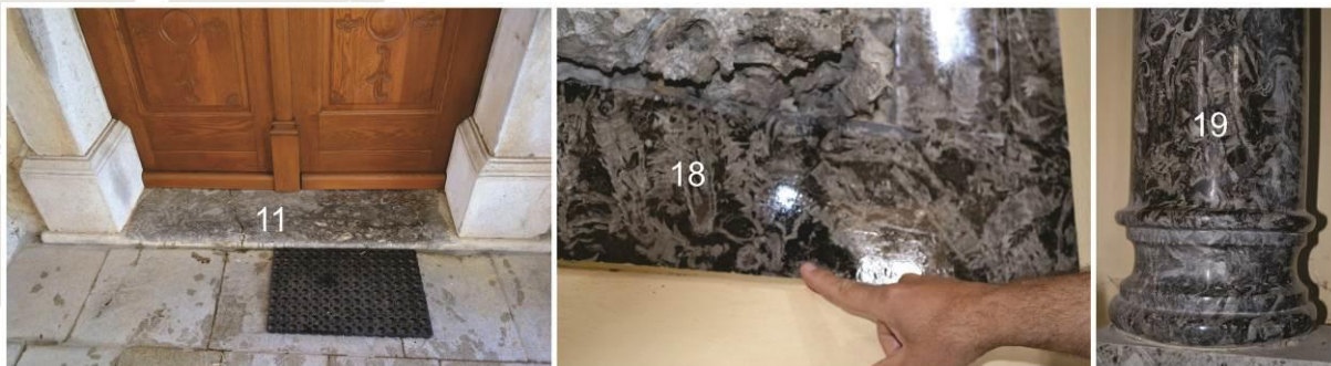
Parts of the building (elements): 11-entrance threshold, 18-edge of Mary statue, 19-Mary altar outer columns
