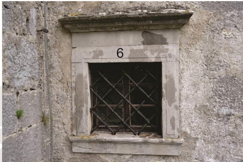
Part of the building (element): 6-window frames (two windows near the main entrance)
