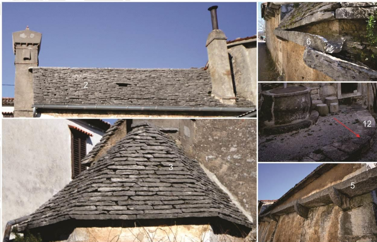
Parts of the building (elements): 2-main roof, 3-extended kitchen roof, 6-eave (gutter) corbels, 6-eaves (gutters), 12-cistern scarp
