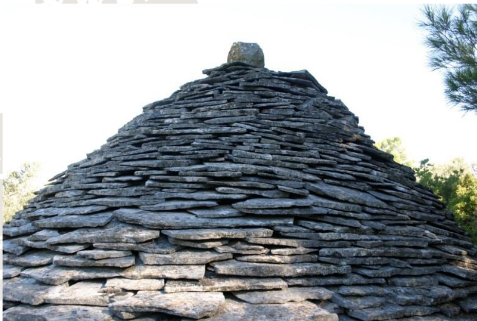
Figure 9: The size and thickness of roof plates downsizes from the edge to the top of the roof. Vrtujak, Korčula, Croatia. Photo: Domen Zupančič.
