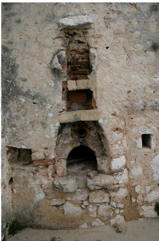
Figure 35: Open fireplace outside of the building. Corbel stone force smoke to detach from the smoke channel. Vidovići, Cres, Croatia. Photo: Domen Zupančič.
