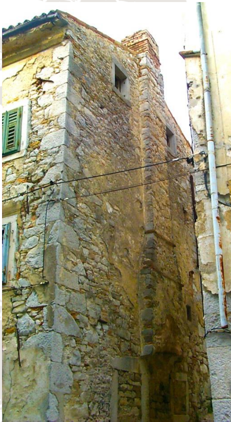
Figure 32: Chimney at the side facade, supported by corbel and arch. The element cross section changes are emphasized using additional horizontal plates. Buzet, Croatia. Photo: Domen Zupančič.
